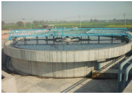
(c) Primary Clarifier
