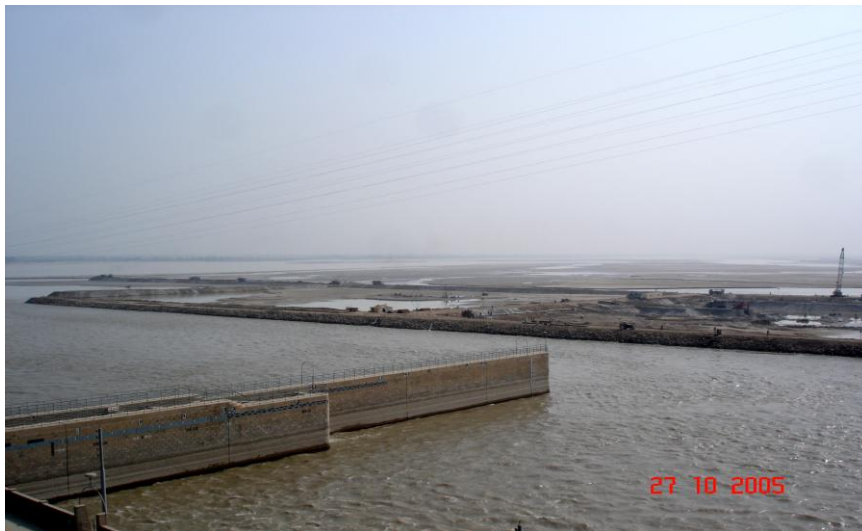
Cofferdams completed in parallel at the front and back of the enclosure
