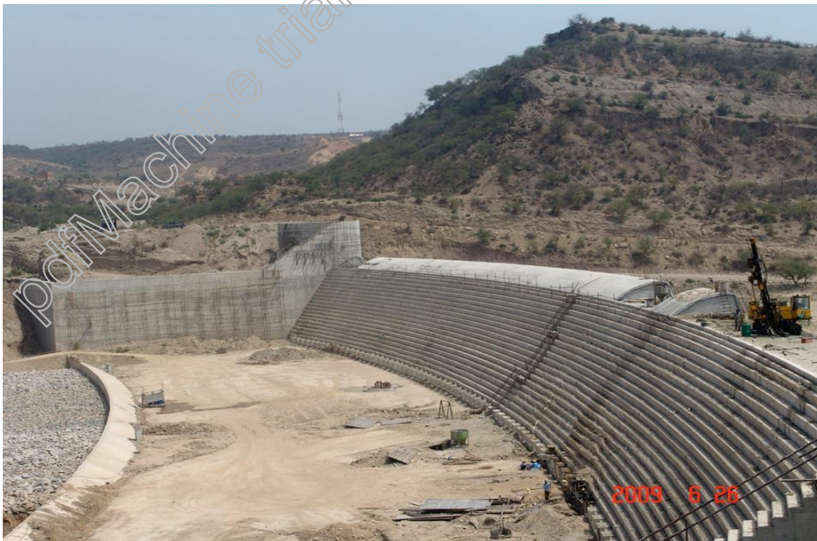
Construction of Control Weir on Upstream of Emergency Spillway is in Progress
