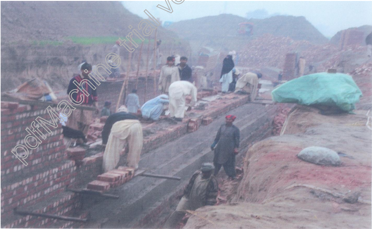
Fig-4: Manual Carrying and placing of Concrete Block on Site in Pakistan
