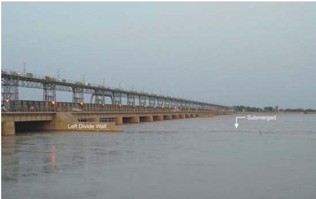
Figure 15: Submergence of Superstructures of the Kotri Barrage
