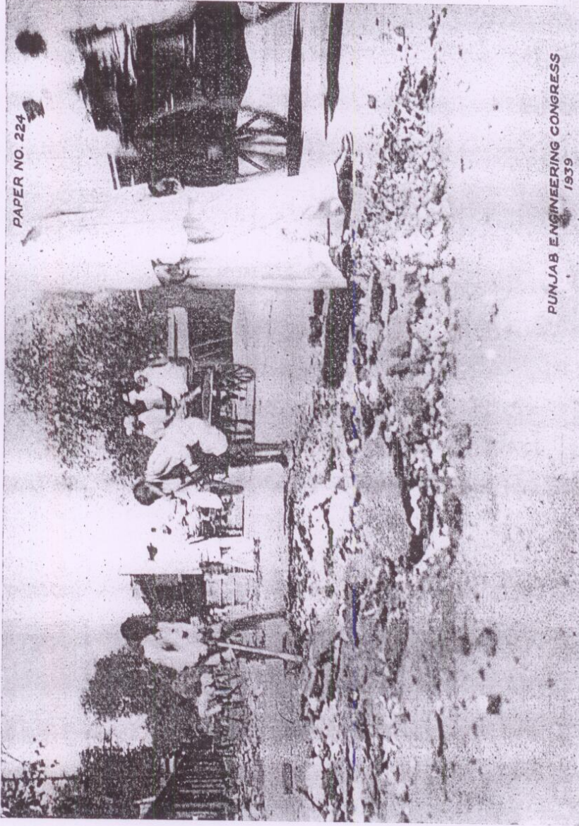
(I) Old Cement-Sandwich Grout Being Dismantled for Laying Cement Concrete, (Concrete Track, G. T. Road.)
