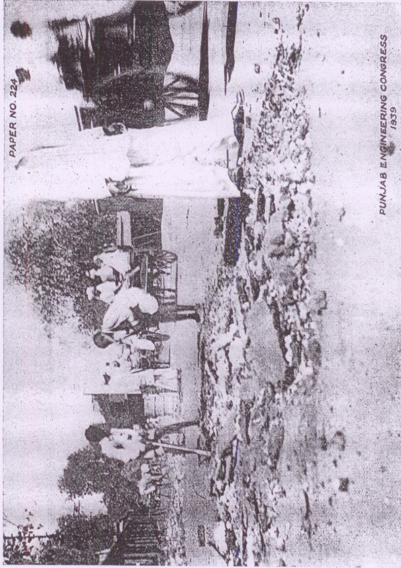
(1) Old Cement-Sandwich Grout Being Dismantled for Laying Cement Concrete, (Concrete Track, G. T. Road.)
