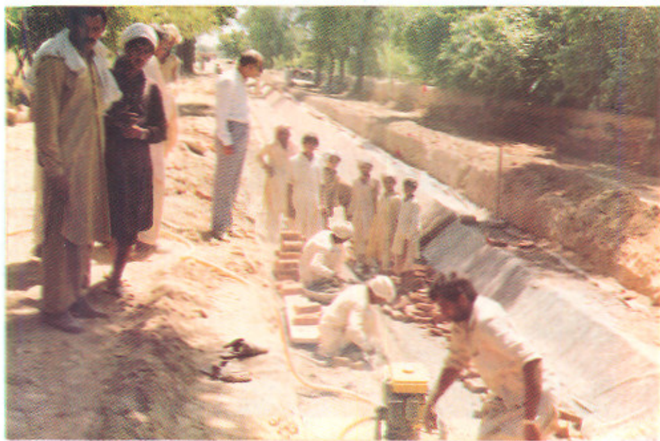
Burried Membrane Lining Comprising Butyle Sheet overlaid by Brick on edge masonry being done in the head reach of Thati Uttar Minor of Niaz Beg Subproject in Punjab.
