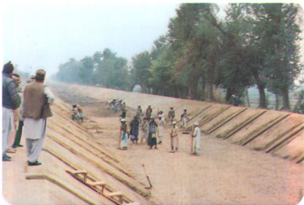
Compaction of Subgrade and Excavation of Profiles along Slope in Progress in 6-R(Hakra) Disty:
