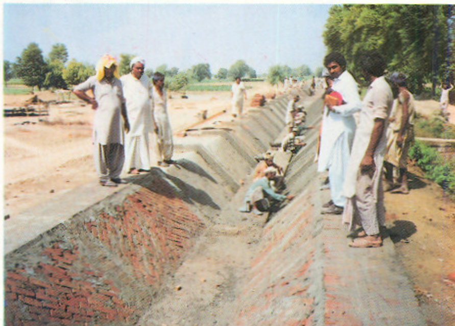
Brick-Masonry and Cement Plaster Lining in progress in the tail reach of 2L|6R minor.
