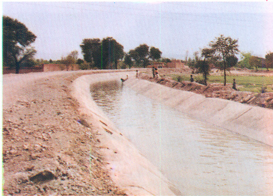
A downstream view of Canal Lining on Warsak lift Canal reach R.D. 59+500 to 61 200
