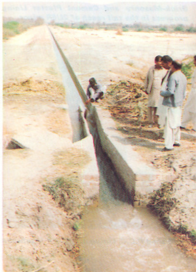
A view of finished rectangular Lined Section U/S of Tail Shahkot Disty:
