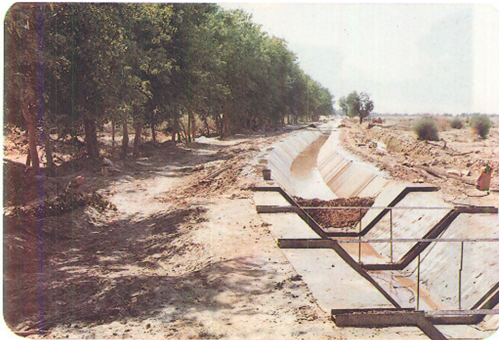
ANOTHER CHANNEL UNDER LINING PROCESS. THE EARTHEN BUND SEEN AT THE END OF THE LINED SECTION IS TO HOLD WATER FOR CURING.
