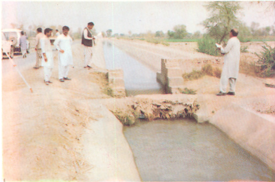
A View of finished R.C.C. Lining of Shahkot Disty: as seen from RD. + 131
