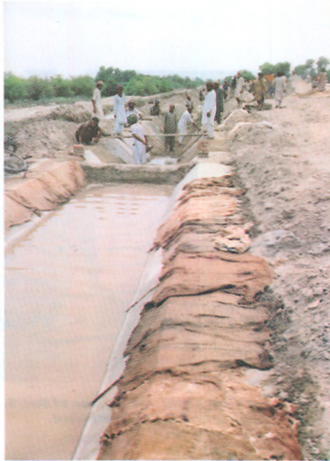
Laying and Curing of P.C.C. Lining along Lundo Minor in Progress at RD.8+000
