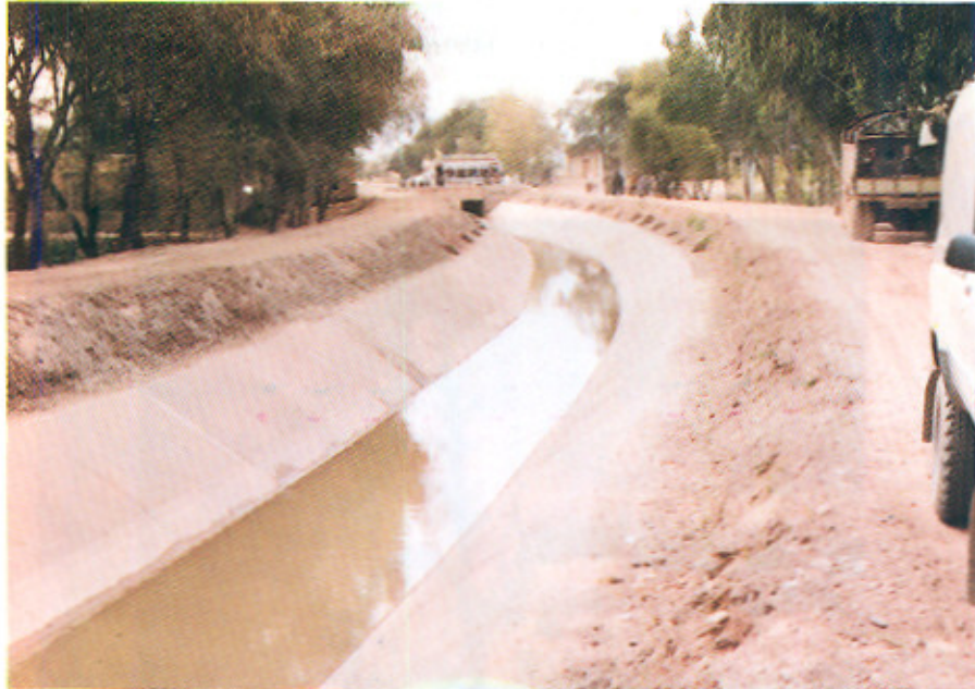
An upstream view of Kohat Road Crossing in the Lined reach of Warsak Lift Canal at R.D. 101+000.
