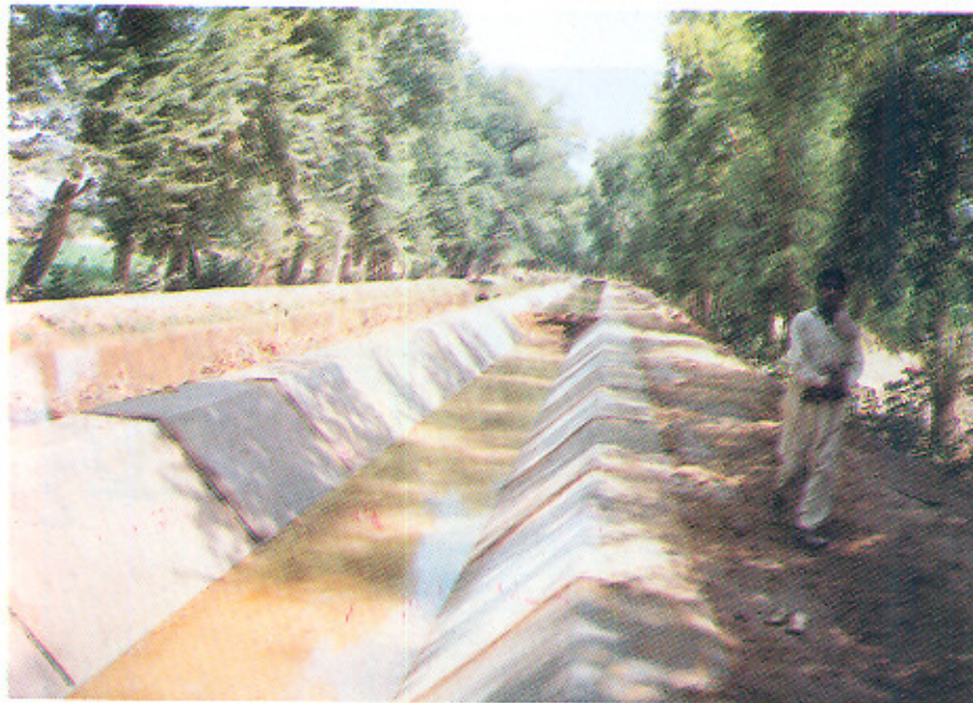
A completed view of P.C.C. Lining on a Channel in Pakpattan Sub-project. The Old Channel can be seen on the left.
