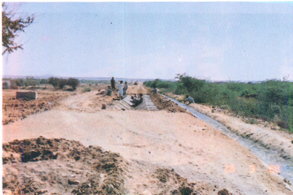
A view of start of P.C.C. Lining in minor No. 3. Existing Minor can be seen on the right.
