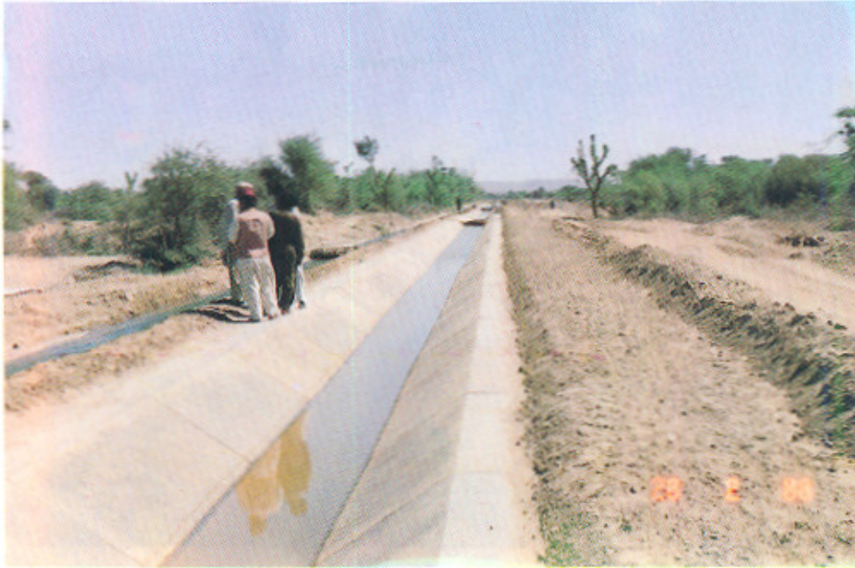
A view of P.C.C. Lining in minor No. 2 near R.D. 1+1000. Existing Minor can be seen on the left.
