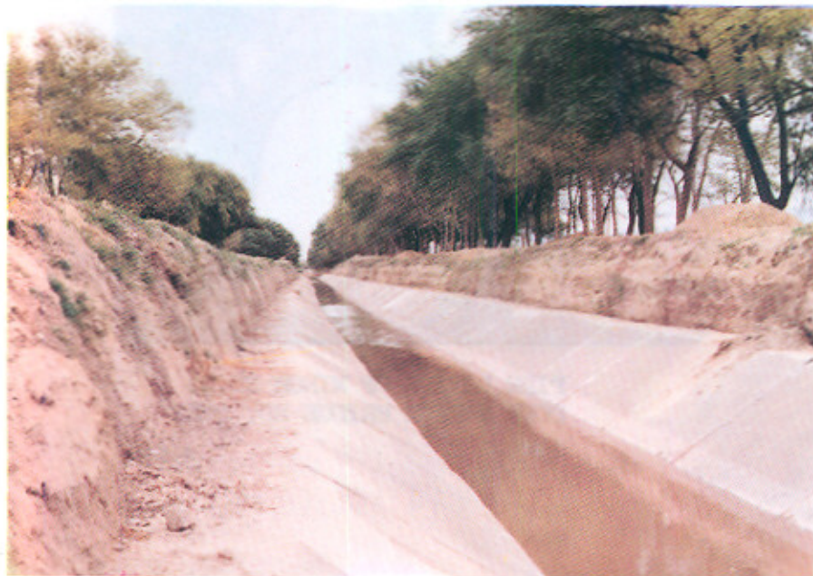
A downstream view of P.C.C. Lining in Warsak Lift Canal R.D. 110+800 to 112+100.
