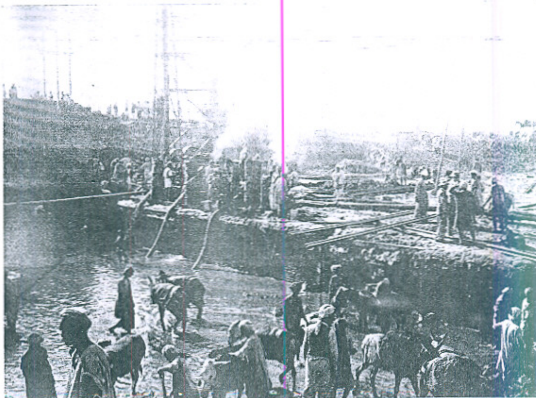
Starting concrete in Bay No. 1 left flank. Mark concentration of local pumping. Date 17-11-36.
