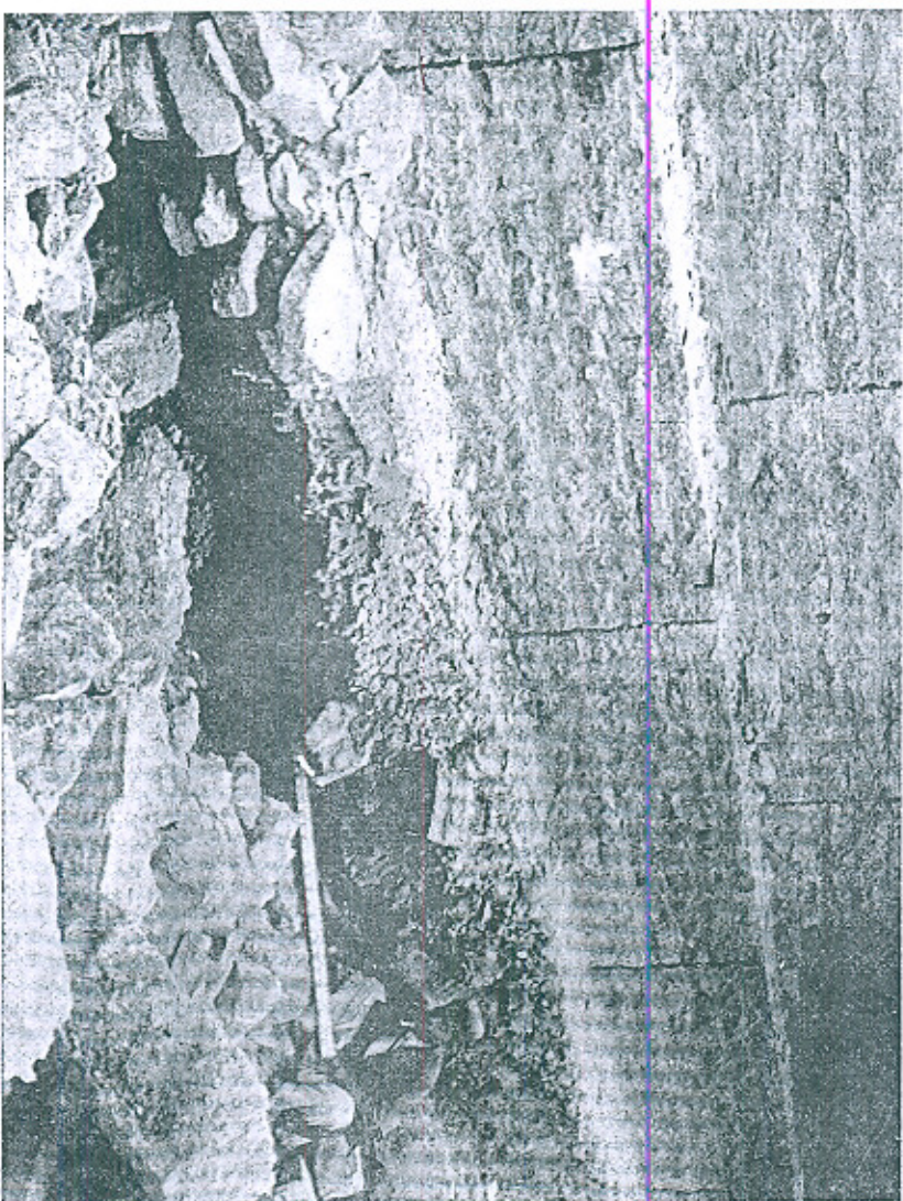
Six feet cavity under Groyne No. 4. Date of photograph. 10-12-36.
