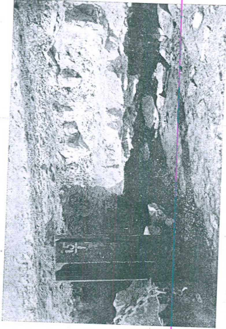
First pile in Bay No. 3 and hollow under old glacis between B and C lines of wells. Nov. 1936.
