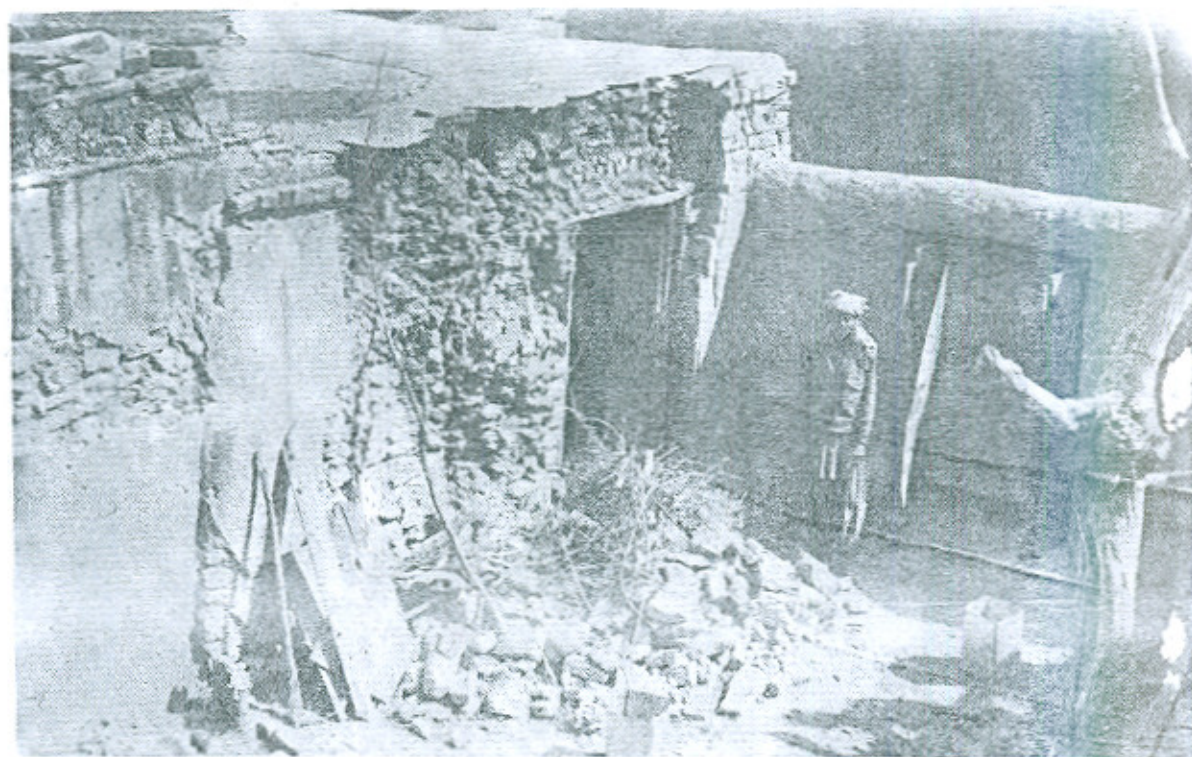
Plate No. 5 Partial collapse of walls of houses built with rubble using mud mortar - K u r i
