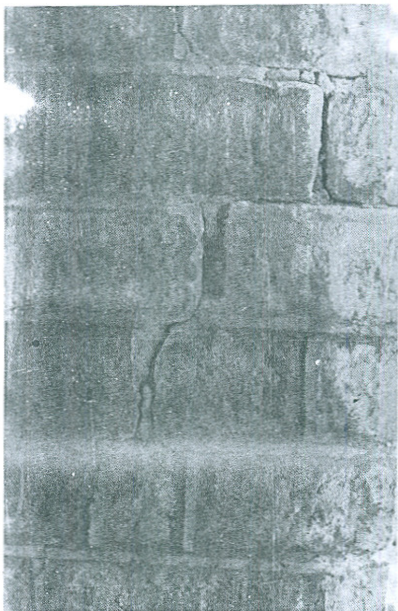
Plate No. 4 Same as Plat-3 Close view of Cracks in Wall
