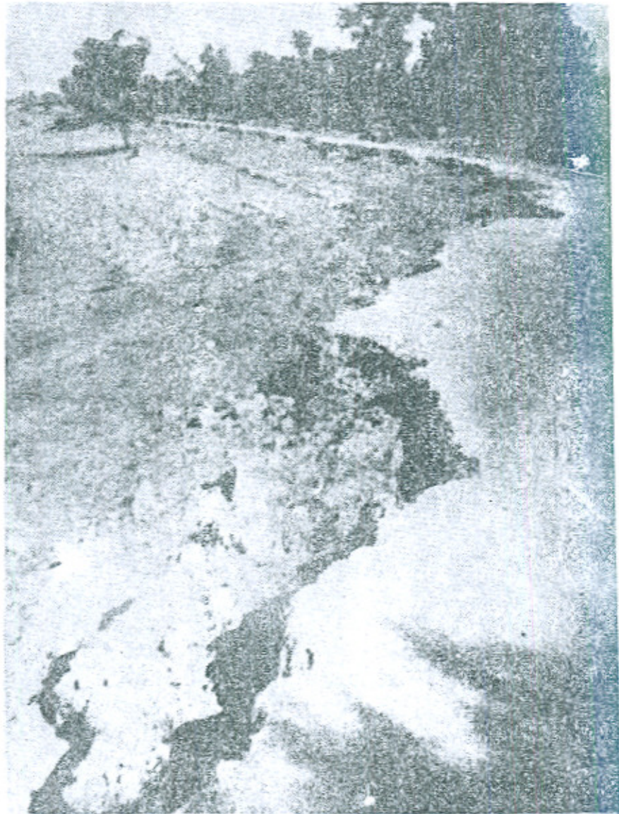
.Chenab Flood Bund after floods 1976. Please note extent of damage and length of beach slope.
