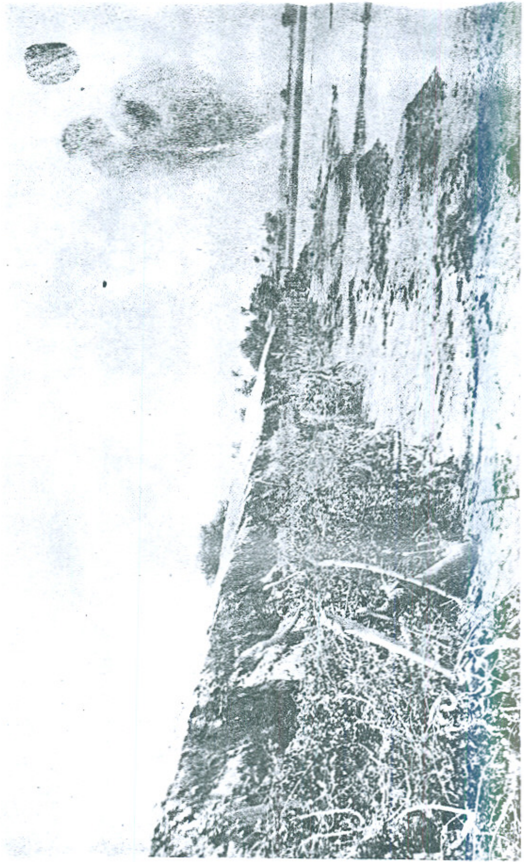
Balochwah Flood Bund R.D.10-11 after Floods 1976. See what it has gone through in spite of permeable Bushing protection
