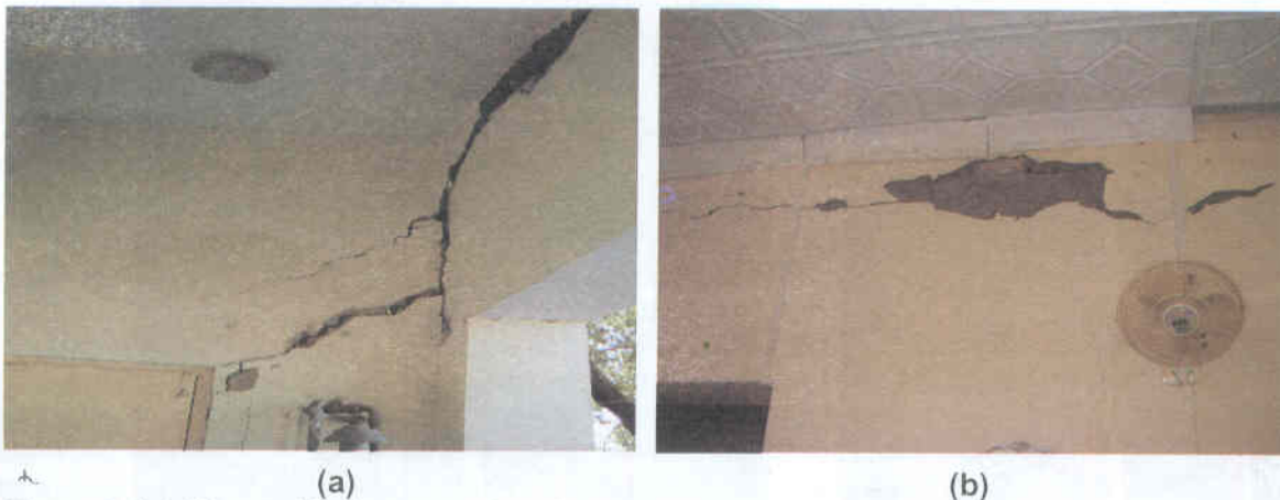
Figure 3: (a) Flexural & shear cracks along with separation of wall from wall connection (b) Shear & flexural cracks along with separation of wall from roof
