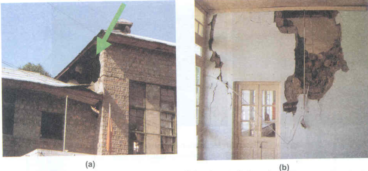
Figure 5: (a) & (b) Collapse of load bearing wall due to out of plane loading
