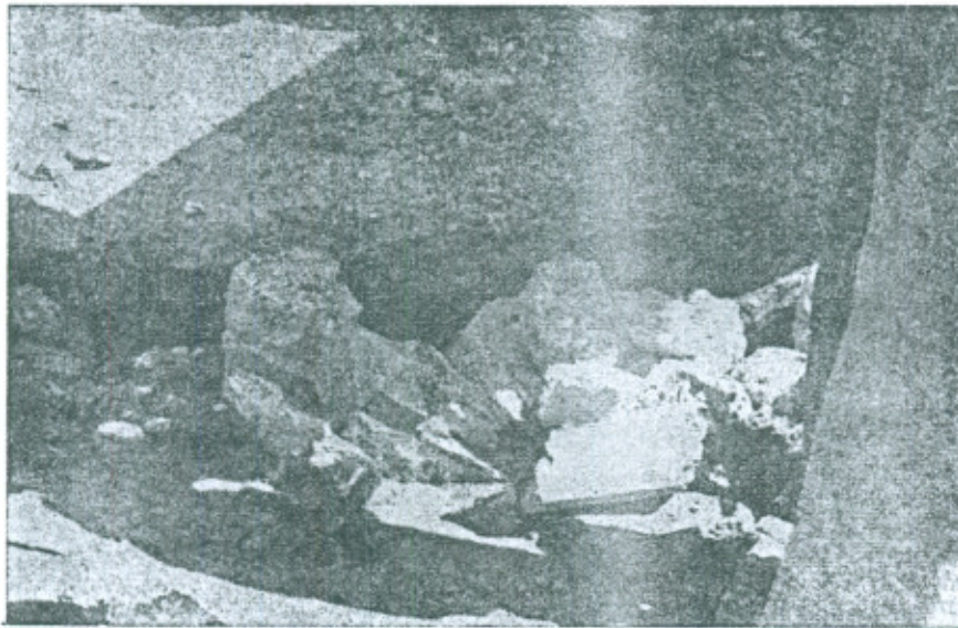
Cavity under the glacis slope.
