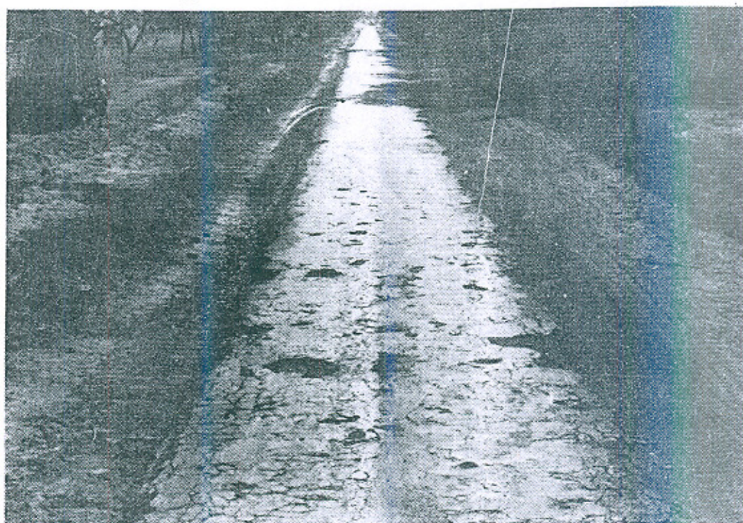
General view of longitudinal cracks and settlement of wheel path
