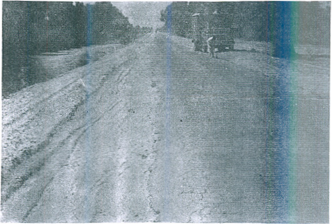
Rapid dis-integration of the edges due to loose dry shoulders
