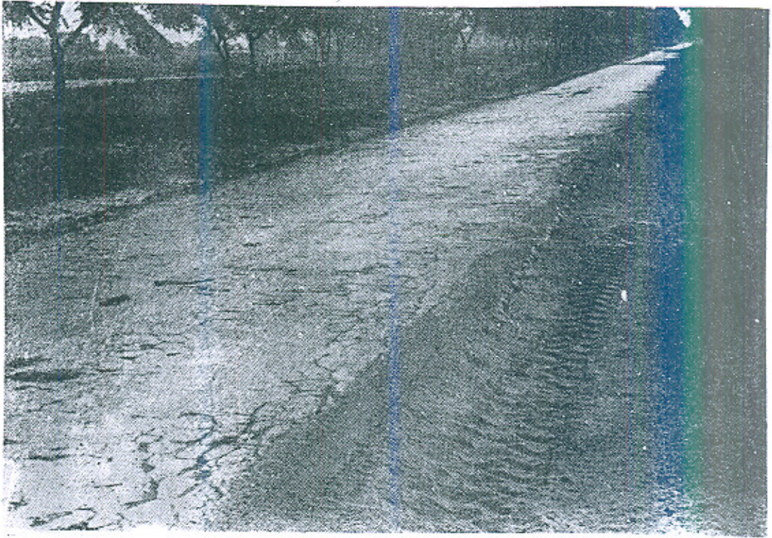
General view of road with pot-holes and eroded dry shoulders
