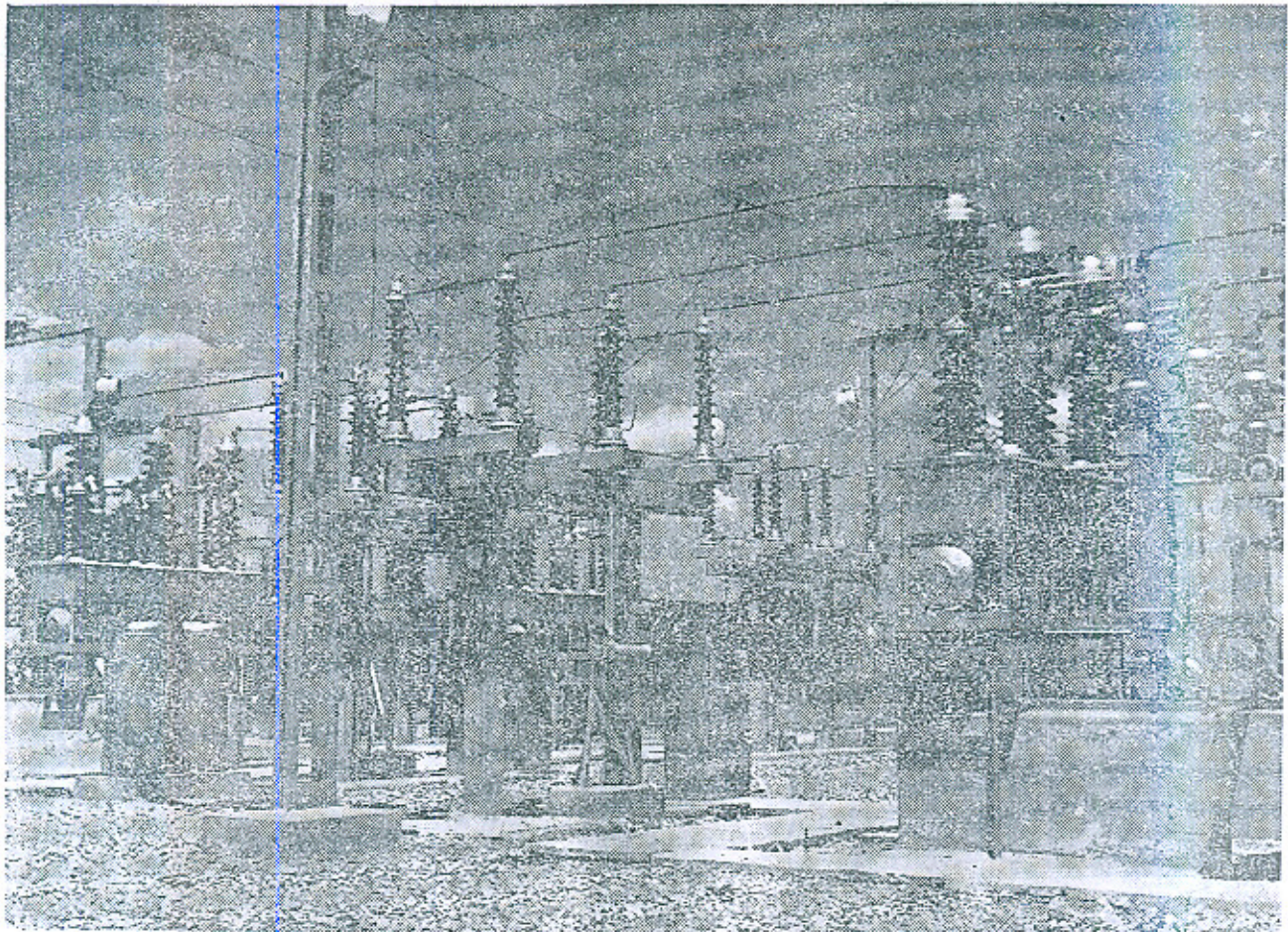
The switchyard at the Chichokimalian Hydel station recently completed
