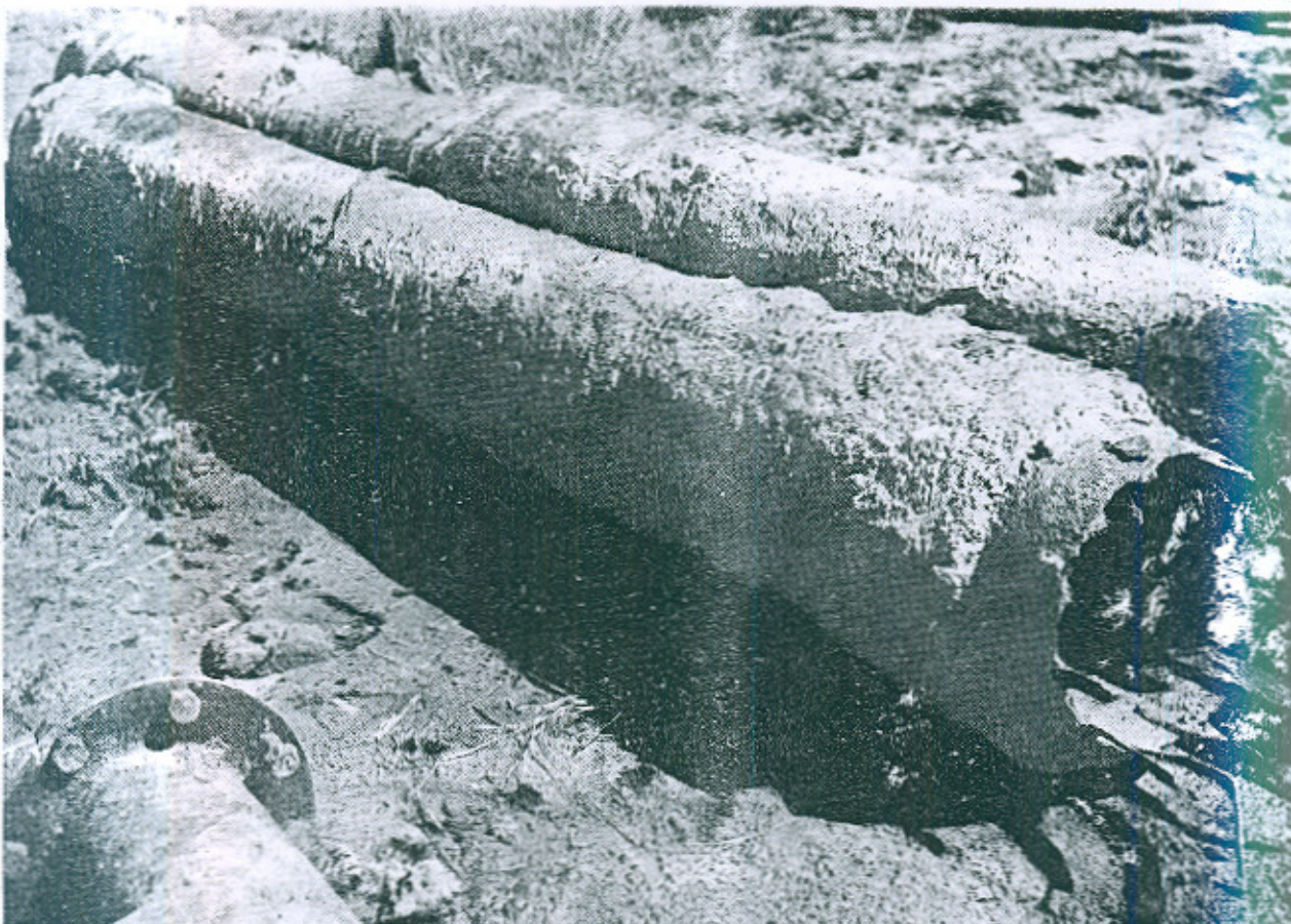
Fig. 3. COIR STRING STRAINER Extracted after 3 years from Gaja Area Groundwater conductivity 20,000 m. mohs/cm.
