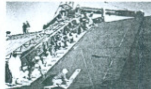
A view of Concrete lining with machine in Chashma Right Bank Irrigation Project Stage-III in Progress
