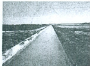
A view of Concrete lined Canal under the Revamping /Rehabilitation of Irrigation and Drainage Systems in Sindh Project
