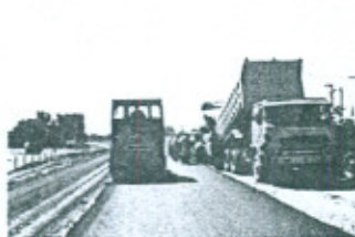
Laying and Compaction of Asphatic Base Course at KM 18+1300 to KM 18+400 Package A of D.G. Khan Rajanpur Road Section
