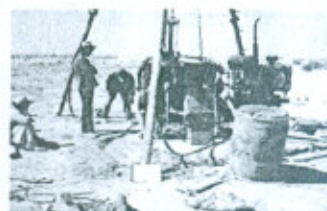
Drilling for Geo-technical Investigations in Progress with Rotary Rig in the Extension of Pat Feeder Canal Project Extension Area.
