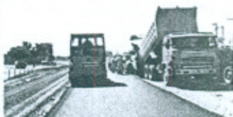
Laying and Compaction of Asphaltic Base Course at KM 18+1300 to KM 18+400 Package A at D.G. Khan Rajanpur Road Section
