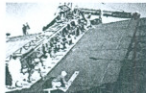
A view of Concrete lining with machine in Chashma Right Bank Irrigation Project Stage-III in Progress
