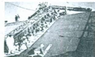
A view of Concrete lining with machine in Chashma Right Bank Irrigation Project Stage-III in Progress
