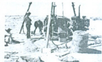
Drilling for Geo-technical Investigations in Progress with Rotary Rig in the Extension of Pat Feeder Canal Project Extension Area.
