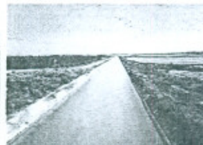
A view of Concrete lined Canal under the Revamping /Rehabilitation of Irrigation and Drainage Systems in Sindh Project
