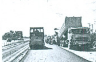
Laying and Compaction of Asphaltic Base Course at KM 18+1300 to KM 18+400 Package A at D.G. Khan Rajanpur Road Section
