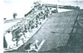
A view of Concrete lining with machine in Chashma Right Bank Irrigation Project Stage-II in Progress
